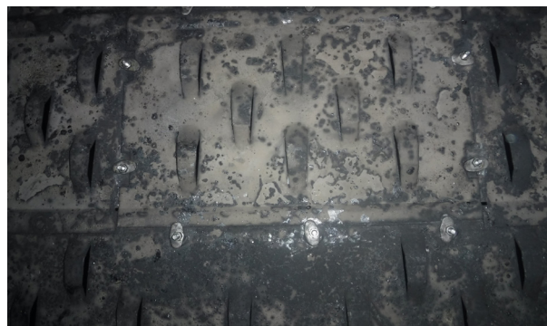
Figure 3. Sulzer XVG™ trays, in tower processing bitumen with sand, after three years of operation.
